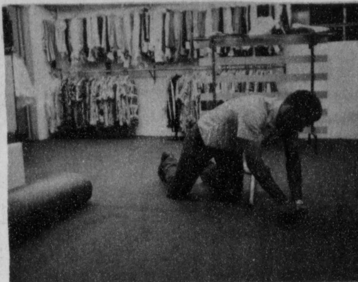
NEW CARPET... Buster Wright installing new carpet in H. L. Davis Department Store, which is a part of the remodeling of the Ladies Department and installation of Refrigerated Air Conditioning.
