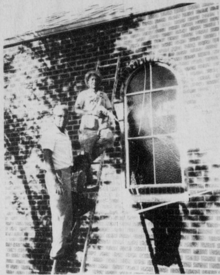
FINISHING TOUCHES; Antonio Yanez at the top of the ladder Aurora Yanez in the middle and Saragosa DeLeon put the finishing touches on the new windows recently installed at St. Joseph's Catholic Church.
