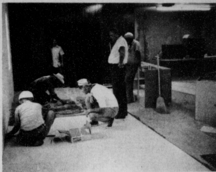
ROBY FIREHALL, Above is a picture of the newly re-modeled Fire Hall Building in Roby. All the work was done by volunteer firemen to include completely re-doing the inside, installing a new ceiling, air conditioning system, new rest rooms, and a new floor. The new building is going to be used as a meeting place for the firemen, a community building, and a site for family reunions. Pictured are Kidd Waddell, Pete Driver, Ruben Rodriguez, Howard Fought, J. M. Whitfill and Wayne Pursley. Plans are to remodel the exterior in the near future.
