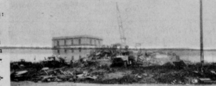
DEMOLISHED COURT HOUSE: Wrecking crews put the finishing touches on the old Fisher County Court House last Monday.
