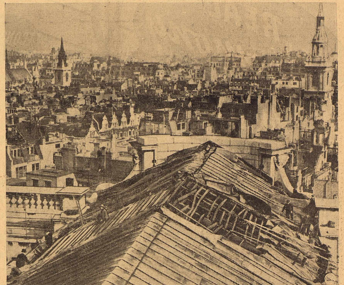
There's construction in war-torn London, as well as destruction. Here workmen are hard at work repairing roof of famed St. Paul's Cathedral where Nazi bombs left gaping hole. It takes twice as many workers to do the job as it normally would, for men at left are "spotters" scanning skies for returning raiders. Note that almost none of buildings in background is damaged.
