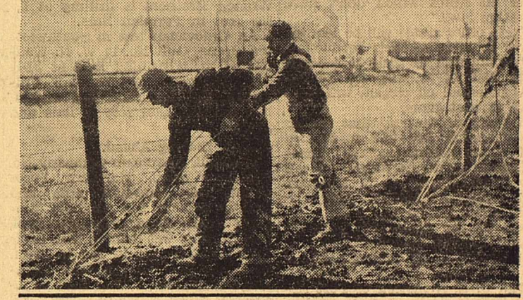
One reason why the giant poles of electric distribution and transmission lines can withstand the terrific strains that they do is because they are securely guyed wherever possible. Here Haskel Wadkins and Wayne Gregston of Midland make secure the guy wires on a transmission line dead-end.
