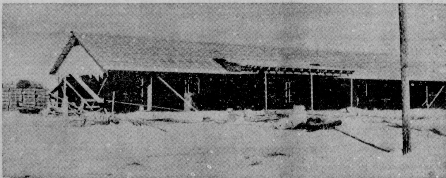
Roof is on and crew working as fast as possible. They have two other jobs scheduled after this one.
