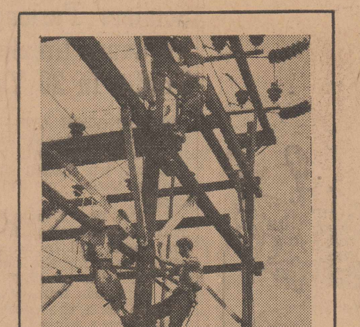
Texas Electric Service workers set a near-record for fast work in building this high-voltage substation to serve Sheppard Field, using emergency stocks of materials already on hand. The substation contains transformer capacity capable of serving the power requirements of an average city of 12,000 population.
