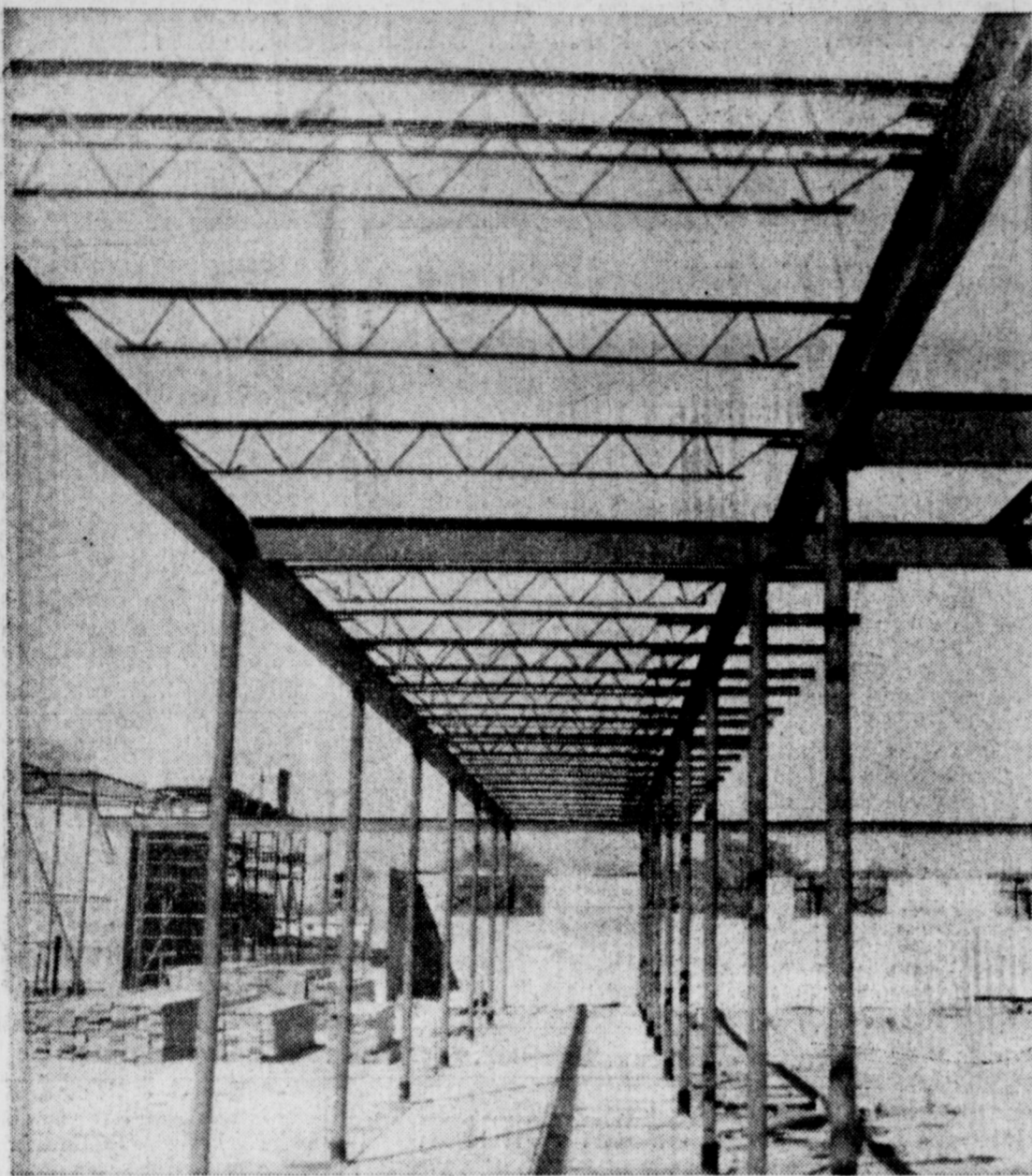
PATTERN IN STEEL -- Construction at Muleshoe's five-project building program is moving along on schedule despite several weeks of cold weather.
