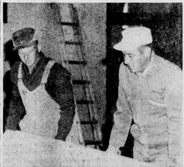
BUILDING RAZED -- Lazbuddie's oldest school building, erected in the '20's, is biting the dust these days to make room for a modern, new structure. Here's Delton Lewellen, who has the contract to raze the building, with his helper Santos Rando, removing one of the partitions. (Journal Photo)
