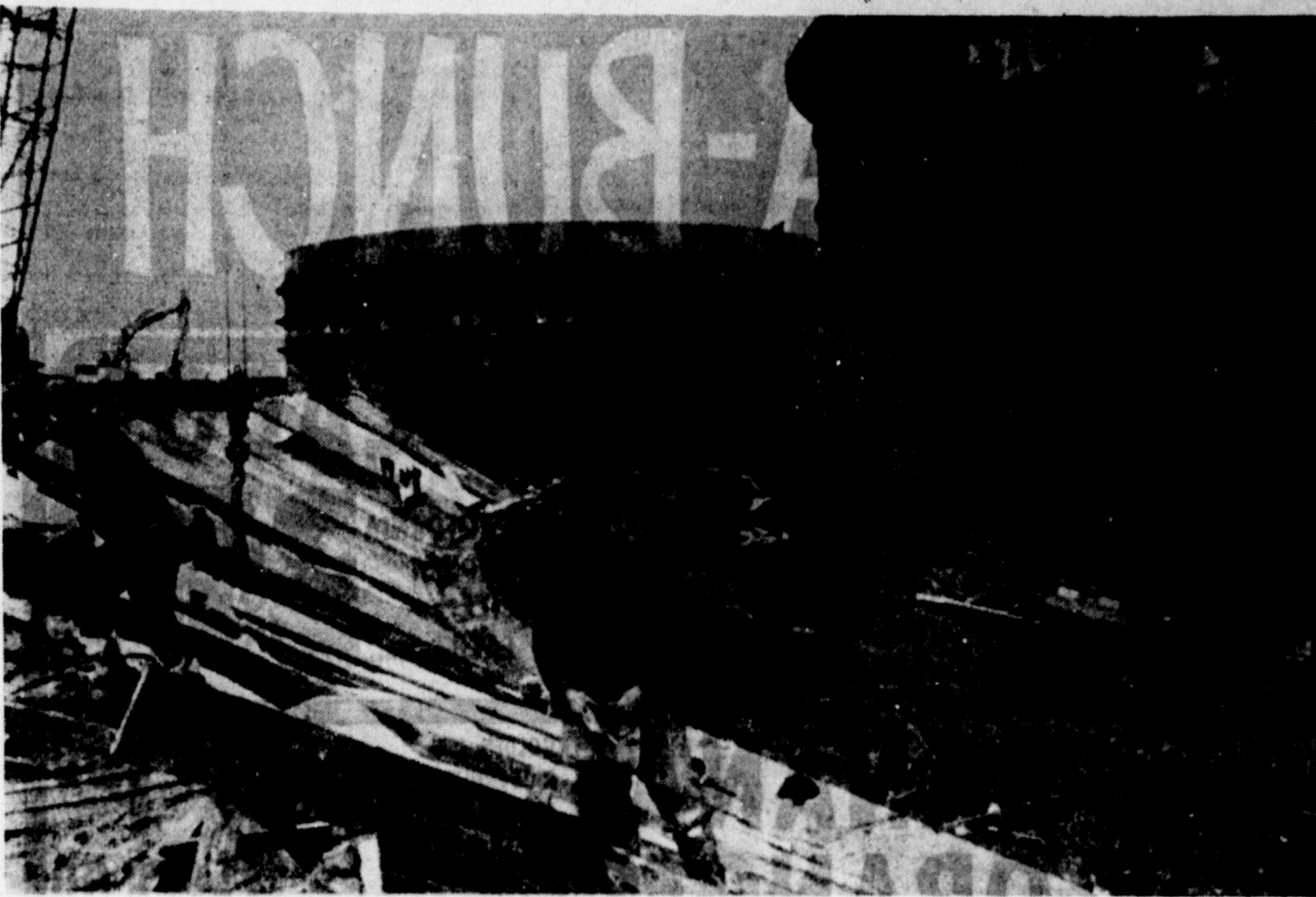
TOP PRIORITY TERMINAL — Workmen emplaced heavy steel panels recently during construction of a massive new oil terminal at Sullom Voe, in Scotland's Shetland Islands. Construction of the terminal, already two years behind schedule, has been given top priority due to its vital role in the overall plan to make Britain self-sufficient in fuel with North Sea production by 1980. (AP Laserphoto)
