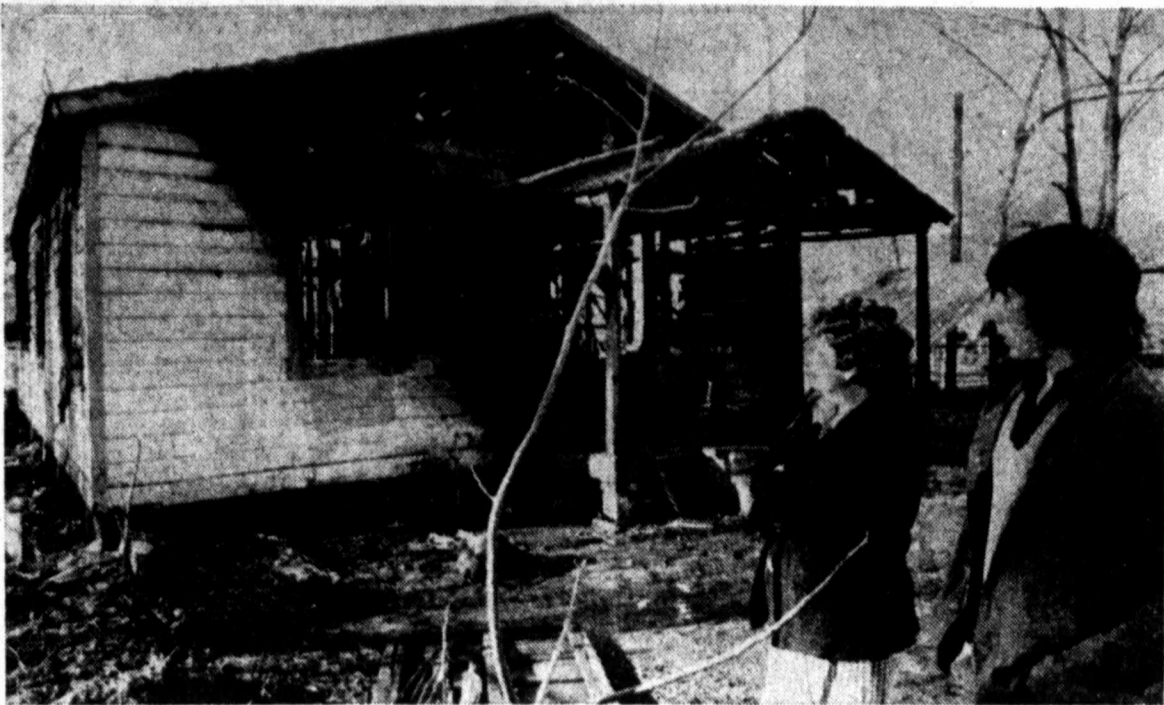
FIVE DIE IN HOUSE FIRE—Nell Slay and her son, Michael, neighbors of the Faustino "Joe" Garcia family, survey the remains of the Garcia house in north Harris County after a fire Sunday night took the lives of Mrs. Garcia and four of the six children, Faustino Jr., 12, Melda, 10, Veronica, 8, and Roxanne. The two children who escaped are John Paul, 13, and Lora, 9. The father was working at the time. The fire was reported to have started when one of the three goats kept on the back porch kicked over a heater. (AP Laserphoto)
