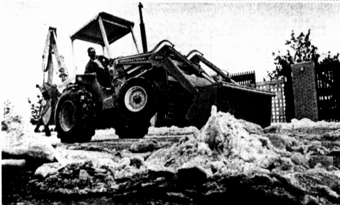
AND A SNOWY HEIGH-HO BULLDOZER — This bucking bulldozer is clearing away ice and remnants of snow in front of the First National-Pioneer Building. The "bull" rider is Glenn Hill. Temperatures rising into the 50s today should give an assist to similar cleanup chores over the city. (Staff Photo by Paul Moseley)
