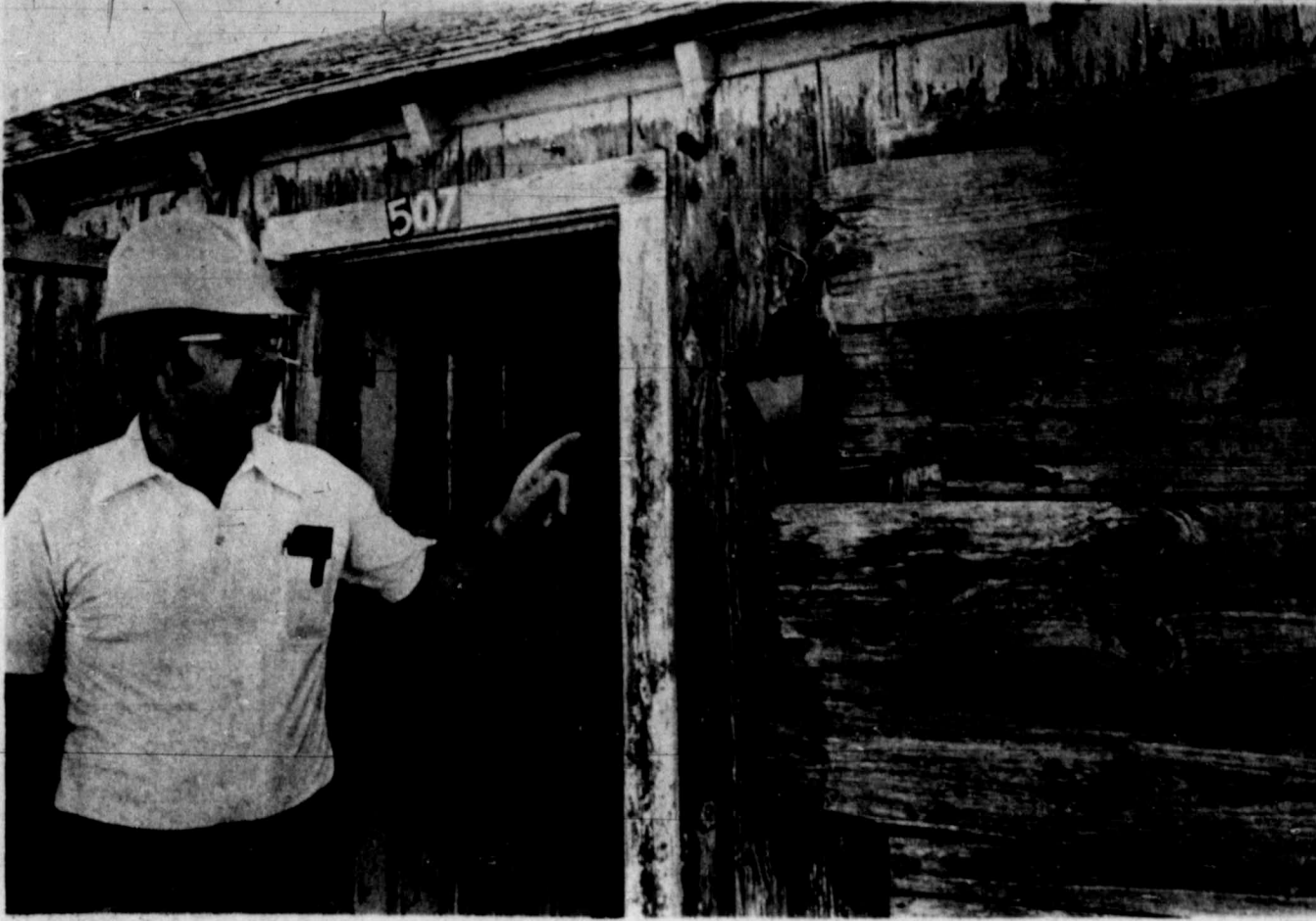
Pointing out a window needing to be replaced at 507 S. Stonewall St. is Bobby Trimble, chairman of
