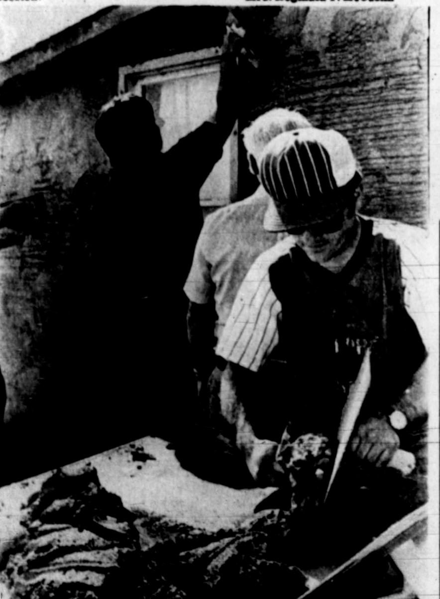
APPLYING STUCCO to the walls of this home at 507 S. Stonewall St. are Terry Claiborne, in hat, and Rocky Valdes. For all the men on this page except Dougherty and Trimble, it is their first time to work on "Christmas."
