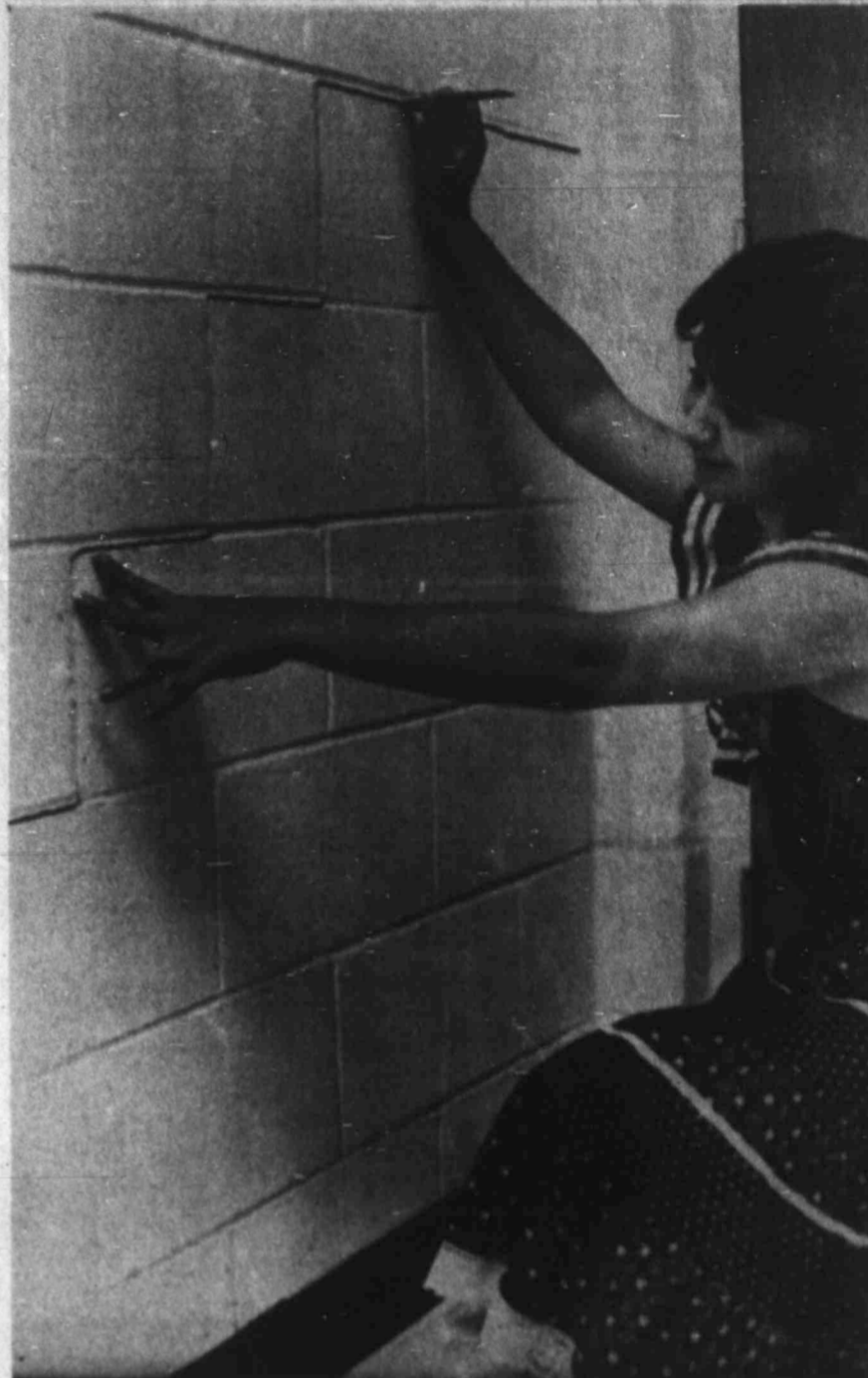
Cracks in the walls of the city municipal building are pointed out by San Juan, Texas city secretary Aracelle Gutierrez. At some points the cracks are large enough for the insertion of a plastic comb. (AP Laserphoto)
