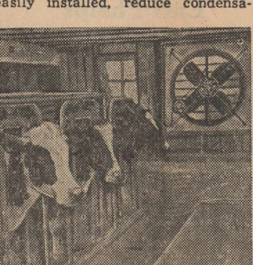
Picture on Vernon Julins farm at Freeport, Ill., shows installation of automatic cooling unit in dairy barn.
