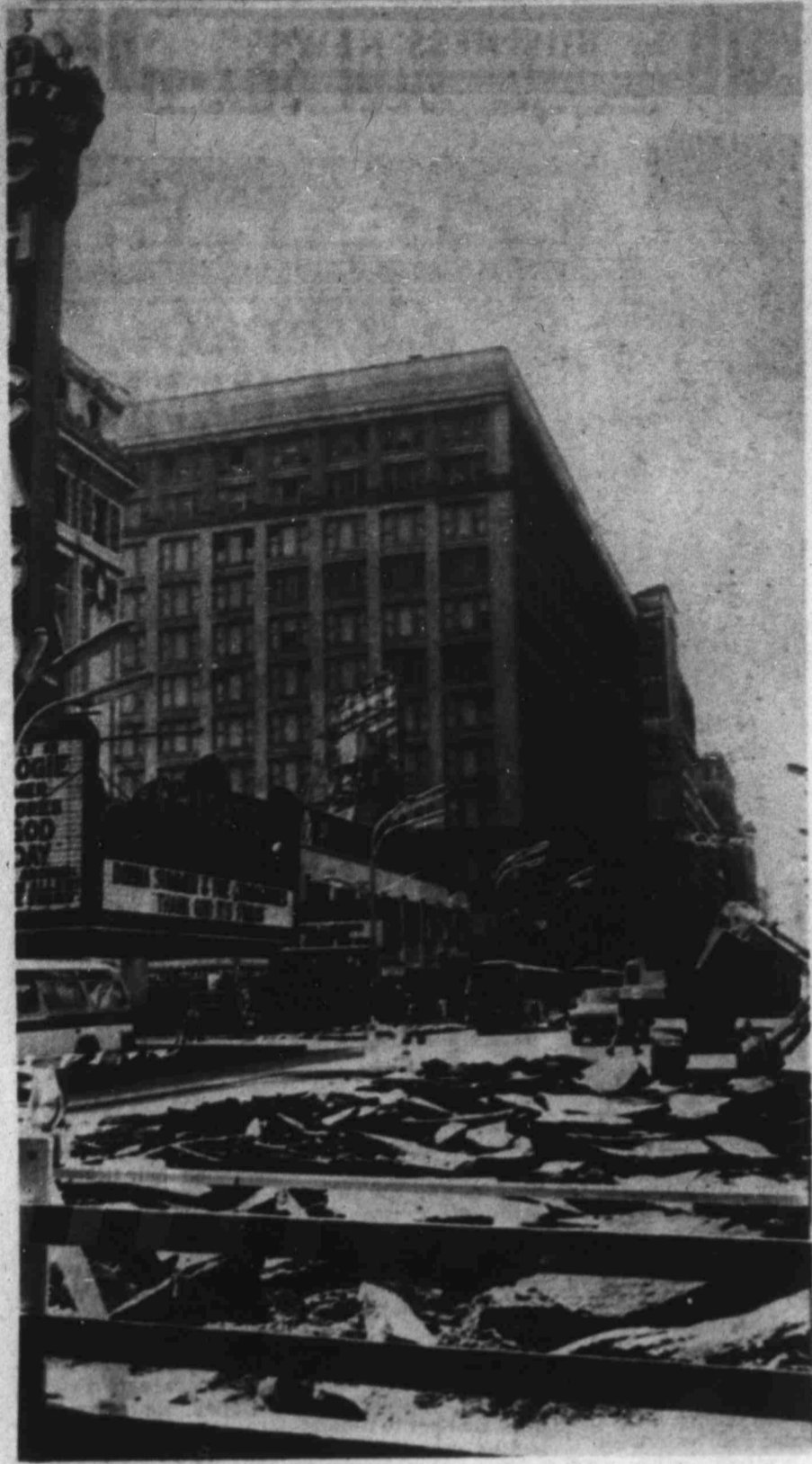
PAVEMENT OF Chicago's famous State Street, that great street, is torn up as work began Monday turning the street into a shopping mall in an effort to revitalize the Loop business district. This view looks south from Lake near the northern end of the mall. Only public transportation will have access to the mall area when completed. (AP Laserphoto)
