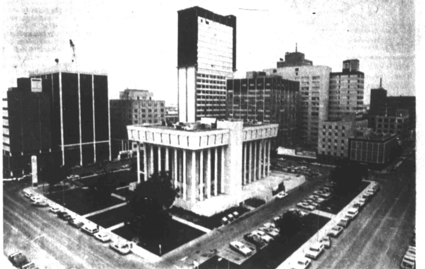
THE DOWNTOWN MIDLAND SKYLINE is enhanced and takes on a big-city look from the vantage point of a high-rise crane 110 feet above the construction site of the 15-story Gibraltar Savings
