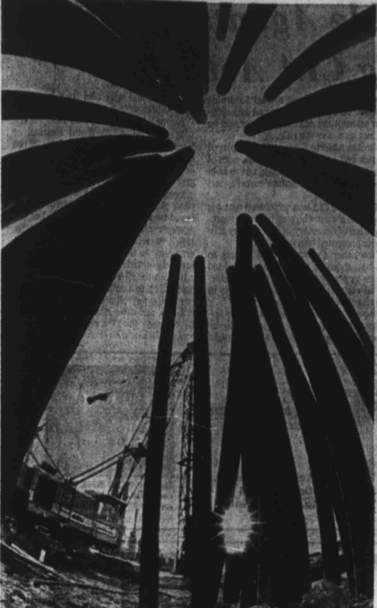
POLE BENDING — A fisheye lens presented this interesting view of pilings being driven into low ground at a Corpus Christi refinery construction site. At the bottom are the pile driver and setting sun. (AP Laserphoto)
