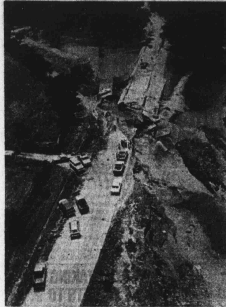
FLOOD ISOLATES CITY — Much of the city of Kerrville is isolated today, following more than 20 inches of rain in the last 48 hours that triggered flash floods. The damaged highway is just one of many roads battered by the torrents which have caused death and destruction in the area. (AP Laserphoto)
