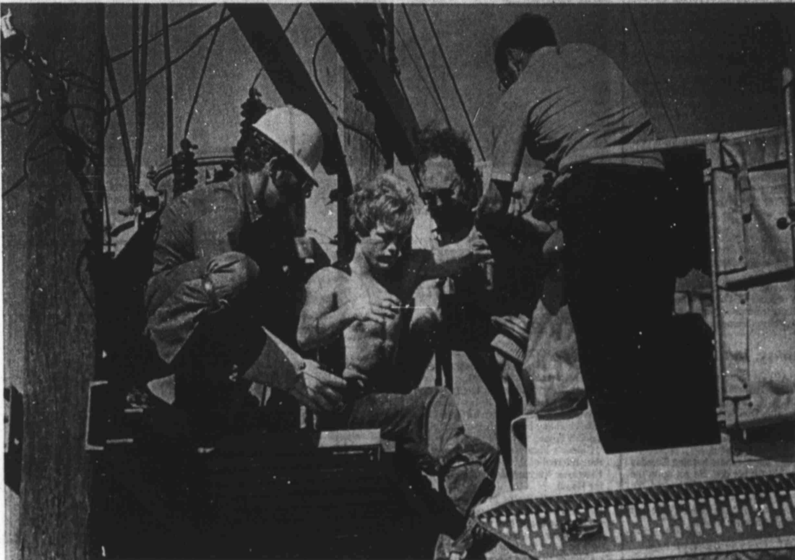
SHOCK VICTIM ATTENDED — Kenny Williams, 20, of 1914 63rd St., receives emergency aid this morning after he suffered an electrical shock while working on a power pole in the 3400 block of Orlando Avenue.
