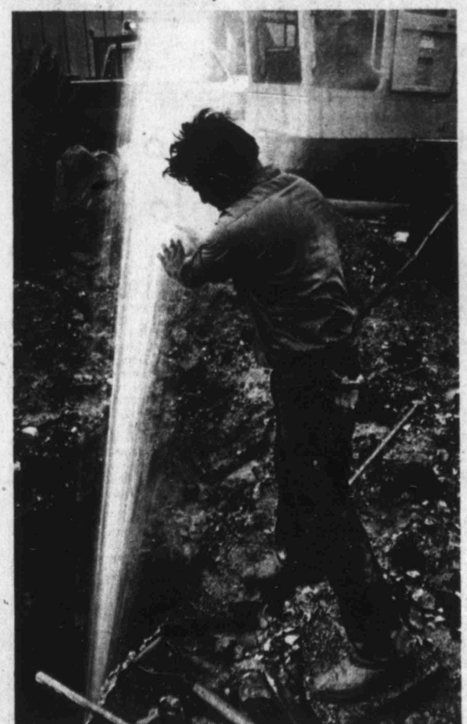
A DRY HOLE It isn't, as a water main at Indiana Avenue and Marienfeld Street comes a gusher after being punctured by a contractor's backhoe about 3 p.m. Monday. City employee Salvador Ramon isn't trying to stop the water with his hands; he's washing them free of mud. It took the city three hours to fix the leak, but at least one Midland outfit didn't mind. Dawson Geophysical Co., 203 S. Marienfeld St., received most of the spray from the 30-foot gusher — and from Monday night's Midland-area showers — on its roof...and on its increasingly green lawn. (Staff Photo)
