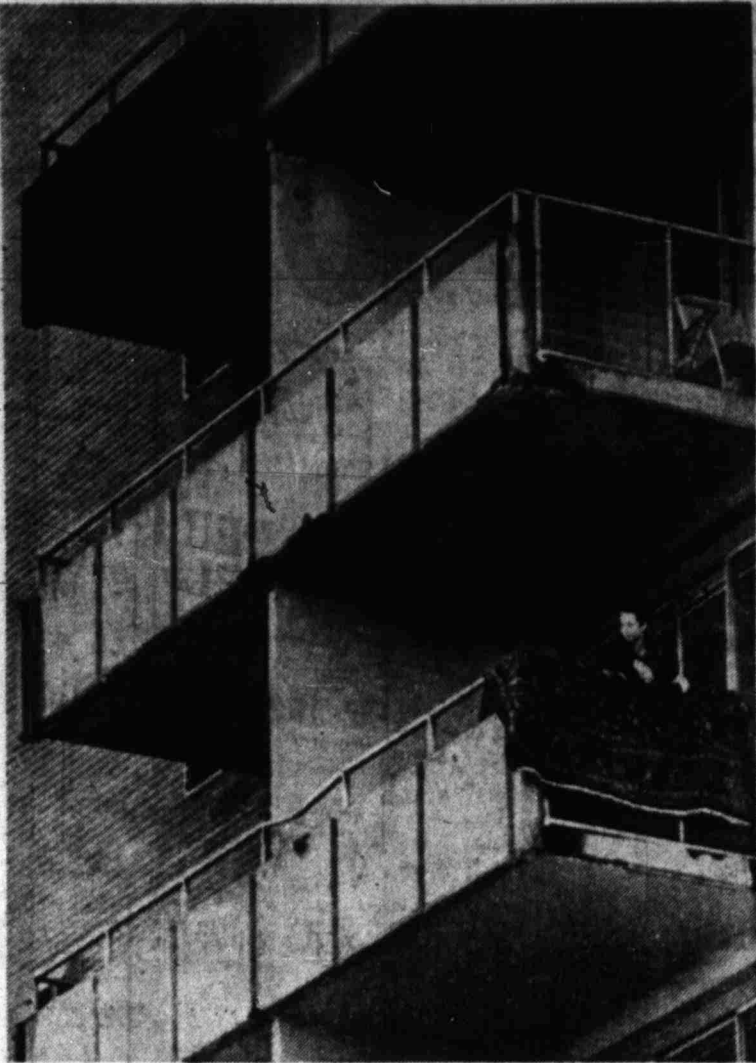
CHECKS FOR DAMAGE — Adrienne Stonek, a resident of Atlanta Towers high-rise apartments, checks her balcony for damage after an early Sunday morning fire forced two residents to jump to their deaths and a third to die in his apartment. Above her is a smoke-damaged balcony on the ninth floor where the fire reportedly began. (AP Laserphoto)
