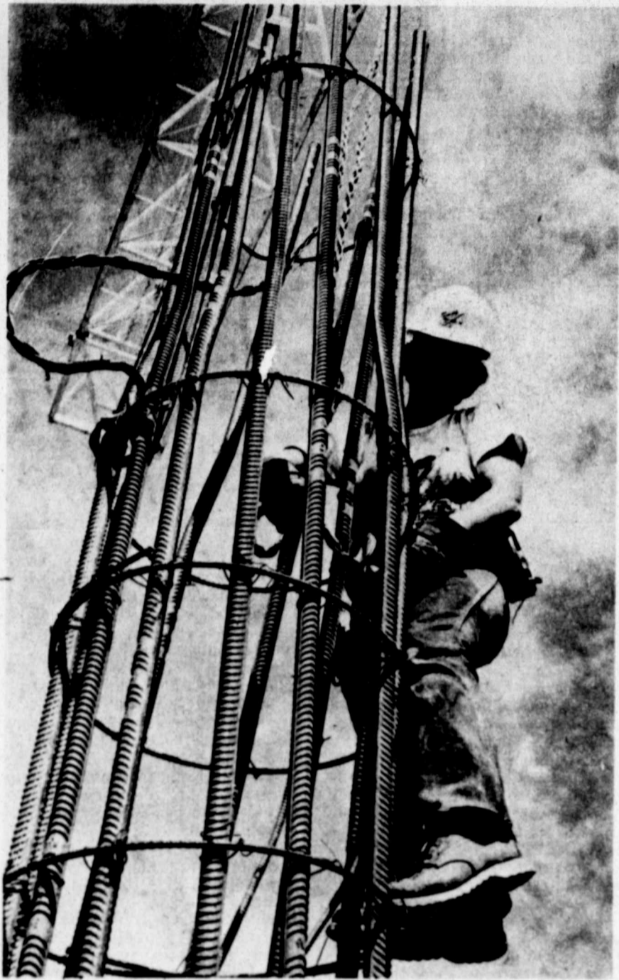
On the job some 30 feet above the ground, Denice Burdick, the first woman ironworker in the Permian Basin, ties off cables for the support columns at the Gibraltar Savings Building in downtown Midland. (Staff photo by Mike Kardos)
