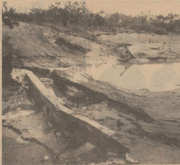
A COUNTY ROAD crossing on the West Kickapoo Creek washed out in 1955 after a 2½ inch rain. Vegetation on the watershed above this crossing was badly damaged by drought and overgrazing. The runoff during this flood was about 10 to 12 ft. deep here at it's peak.
