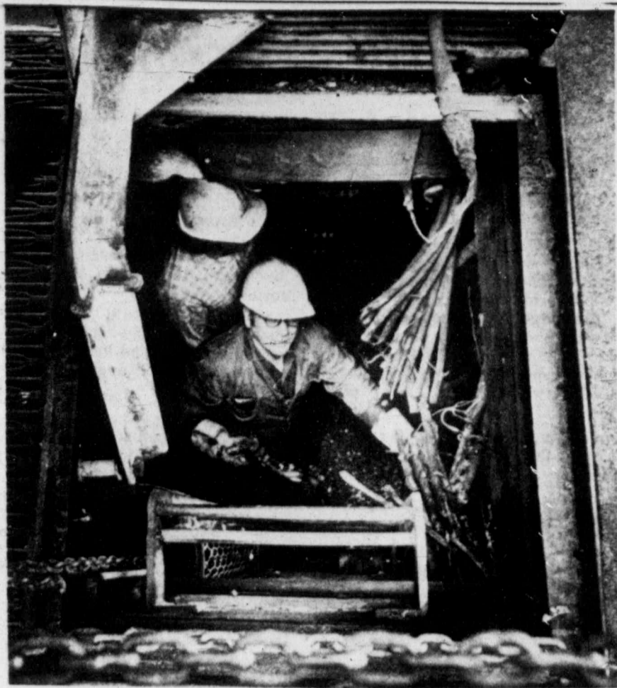
Boston Edison Company workers inside blasted manhole in downtown Boston Tuesday are trying to repair the damage caused after explosions and fires erupted. (AP Laserphoto)
