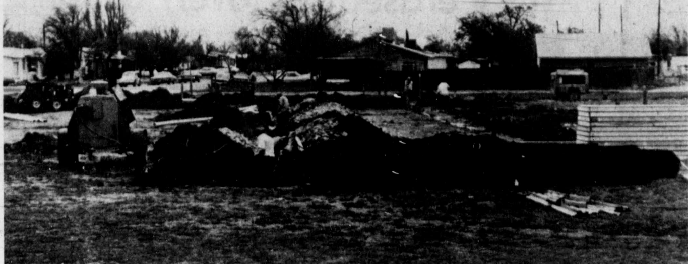
Construction recently began on the Salvation Army's Mabee Westside Corps Center, scheduled for completion this fall, at Holly Drive and Park Lane. The 10,897-square-foot Midland facility will
