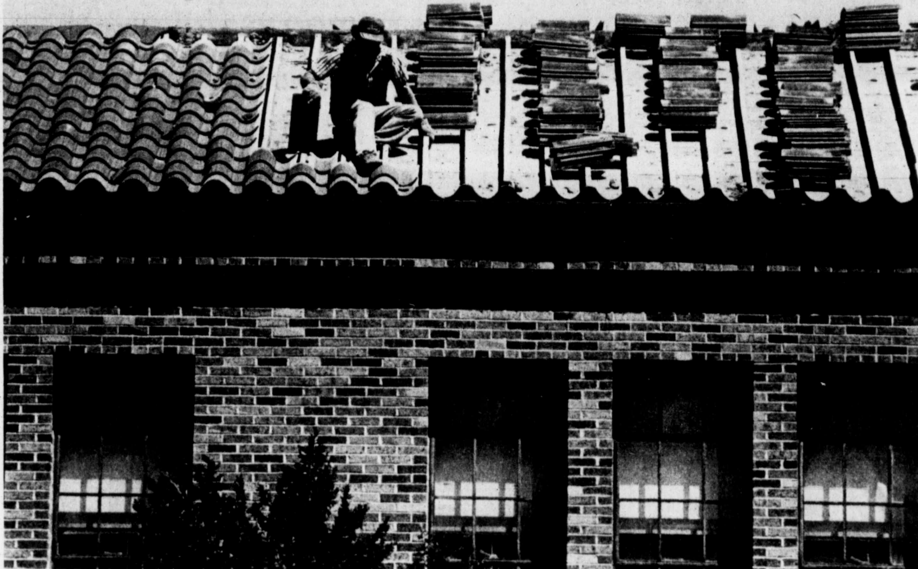
Midland's first school building may soon be nothing more than memories for many, once crews have finished removing reusable materials. Florento Ortega carefully stacks roofing tiles that will be shipped near Bryne, Texas, to roof another building. Built in 1937 for a now-paltry $84,000, the structure served the Midland Independent School District until January of this year, when a Midland bank purchased it. (Staff Photo by Mike Kardos)
