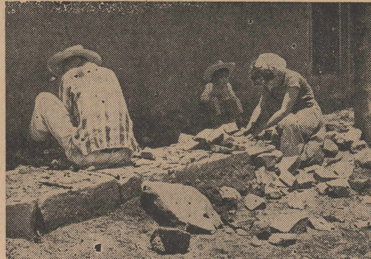
DO-IT-YOURSELF PROJECT ... Family in Tsintzuntzan, Mexico, constructs a sidewalk outside their home. Home improvement project is part of a rural social welfare program of the Mexican government.
