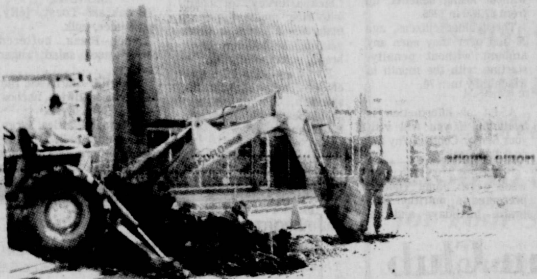
City of Cisco crews are shown working on a water leak located in the 700 block of Conrad Hilton on Wednesday of last week. The water line blew out again Friday morning spraying the sidewalk in front of Austin's Furniture with water. The city crew was back out there by 7:00 a.m. Friday working to repair the leak. (Staff Photo)
