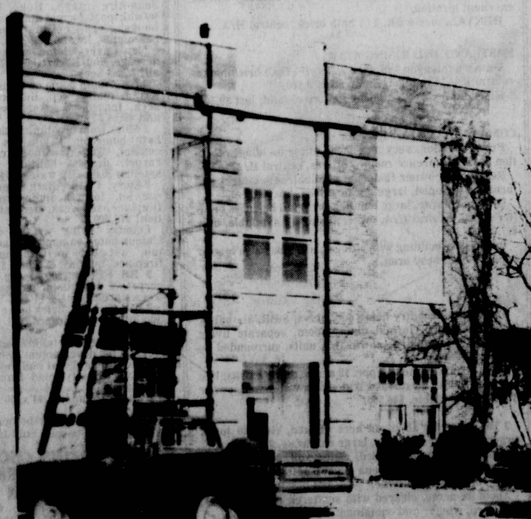
REMODELING CITY HALL will give the building a new and different look. Workers were busy last week giving the old building a facelift. (Staff Photo)
