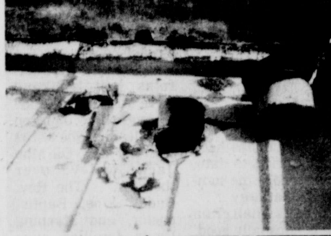
Hole In Roof Through Which Jennings Escaped
