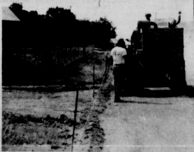
Crews were preparing Front Street Friday morning for the curbing and gutters which will have to be laid before the paving of the street itself. (staff photo)
