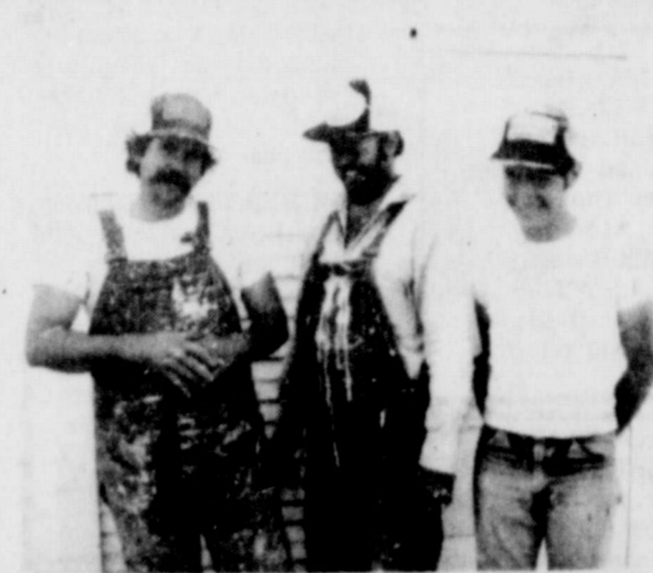
Randy Taylor, Charlie Cole and Greg Swindle assisted in putting new ceiling at City Library.
