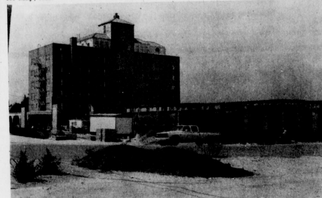
NEW BANK FROM the back side -The above picture, made from the rear of the new First National Bank building, shows that steel for roof and frame work was in place and that the brick work was well underway. The building, about a month behind schedule due to bad weather, is due to be completed about Nov. 1. The picture was made Tuesday. (Staff Photo)
