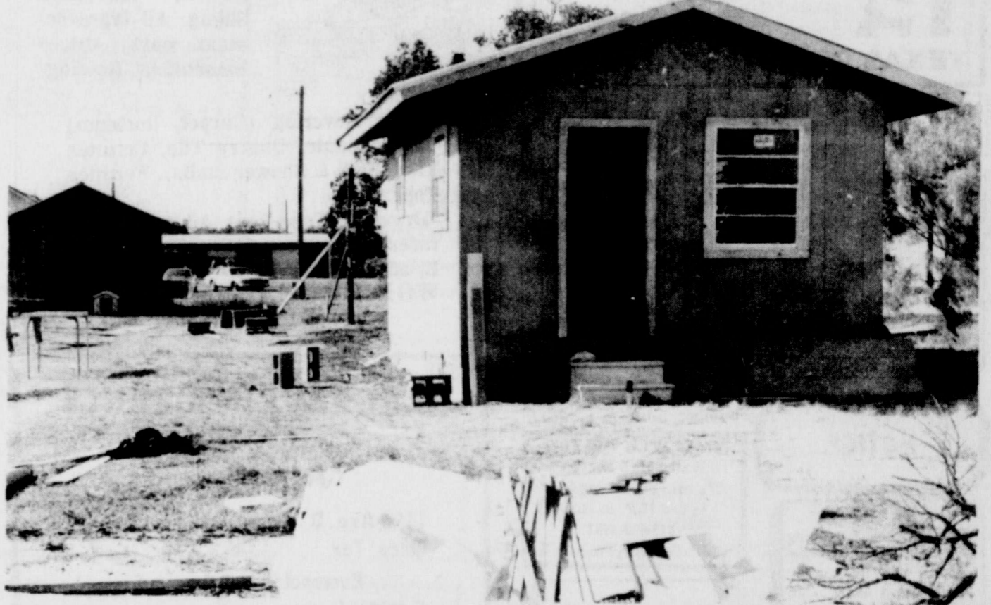
A NEW HOME was built last Saturday for Floyd Crafts of Cisco by the Christmas in May project of the Cisco Chamber of Commerce. In the above picture of the new home, a garage can be seen in the background where Mr. Crafts has been living. (staff photo)
