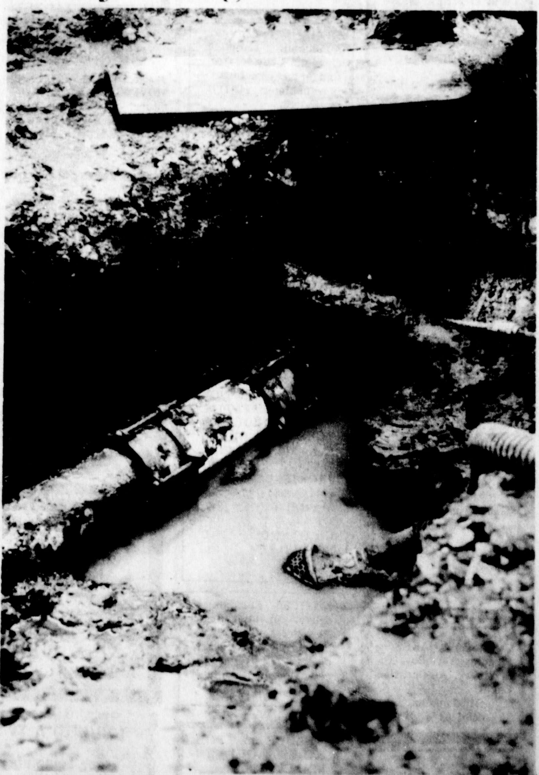
NOW IT'S FIXED — A water leak in the alley near Lobo and J.R.'s was hopefully permanently repaired Monday since an old leaded hub was cut out and replaced with a dresser coupling, according to City Manager Mike Moore. Mr. Moore said he was told the leak had been repaired almost every year for the past ten years whenever the soil changed with the weather. He said Cisco is experiencing some water leaks again this year, due to freezing weather, but it is not anywhere near the major condition of leaks last winter. (staff photo)
