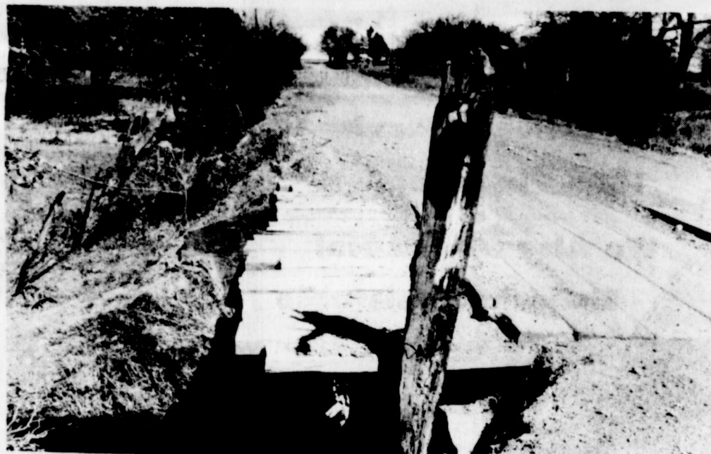
This photograph shows the bridge referred to by Danny Schaefer in his report to the County Commissioners. It is located between the Danny Schaefer and Claude Harris property south of Cisco. The photograph was made Feb. 11.
