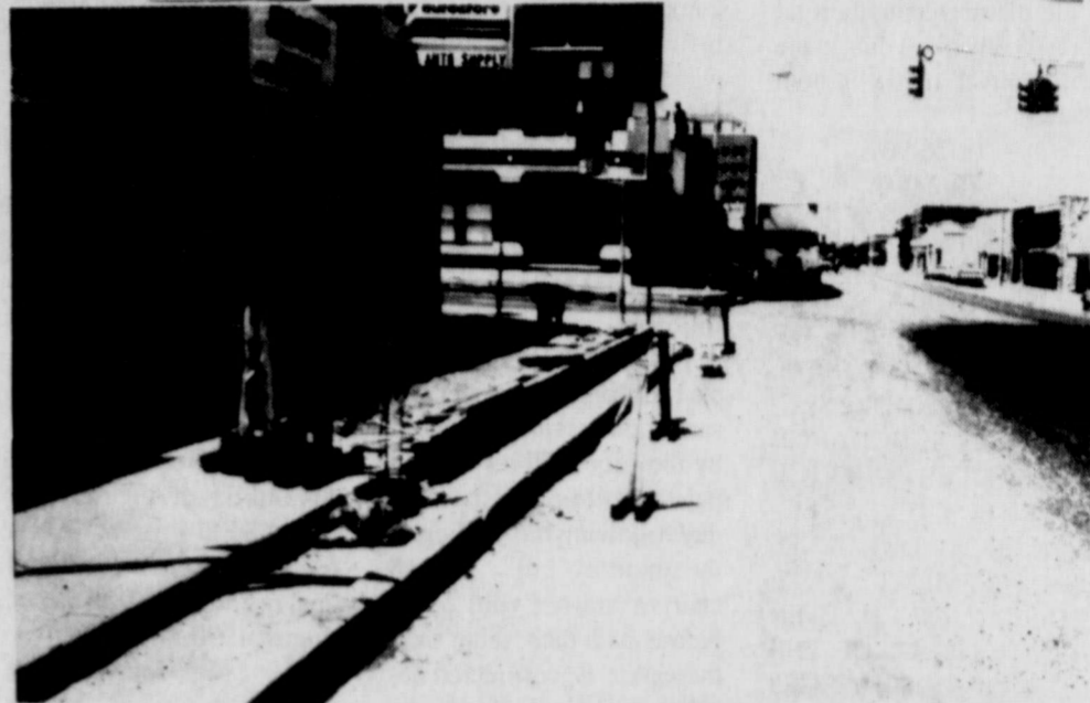
SIDEWALK REPAIRS-- Workers were busy last week repairing damaged sidewalks at the intersection of Conrad Hilton Avenue and Sixth Street. The sidewalks were damaged in June when a 19-axle tractor-trailer attempted to make a wide right turn from Conrad Hilton onto East 6th Street. The sidewalk in front of Dixon's Auto Supply and beside Reynolds Mfg. Co. were crushed under the weight of the truck. (Staff Photo)
