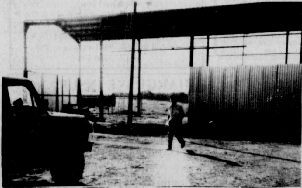
Workmen are beginning to put metal siding around the frame of a large new manufacturing area at Texas Custom Fabrications Inc. This complex is located on Highway 183 just Northeast of Cisco.
