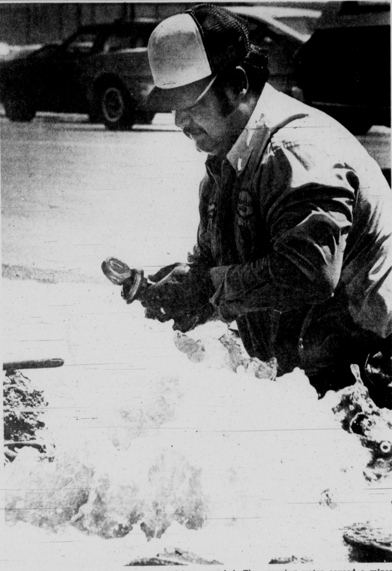
Several members of a city crew tried for more than 30 minutes Tuesday to replace a worn-out water valve in a main in the 100 block of East Illinois Avenue before Raymond Martinez, 30, succeeded.
