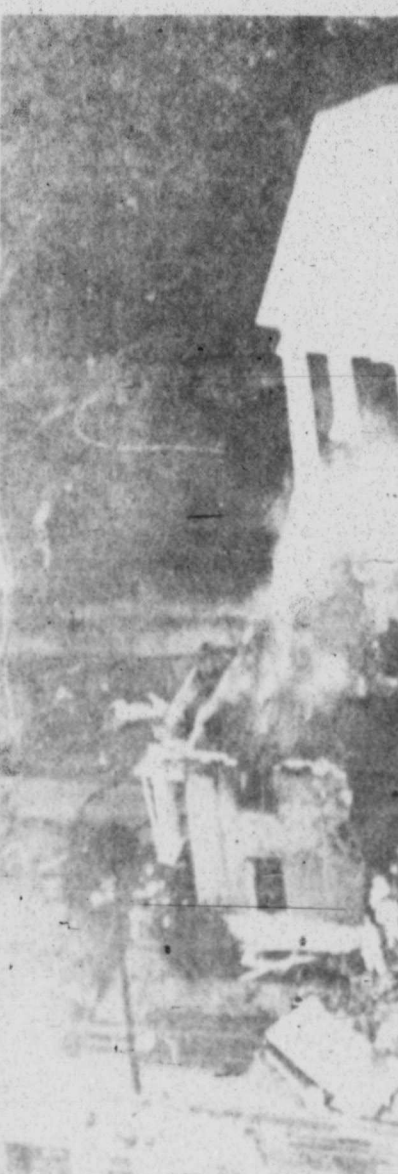
The smoking ruins are all that remain of the Greene County Office Building, foreground, and historic county courthouse in Stanardsville, Va. An explosion, caused when a backhoe ruptured a gasoline tank, rocked the buildings Wednesday, injuring 15. (AP Laserphotos)
