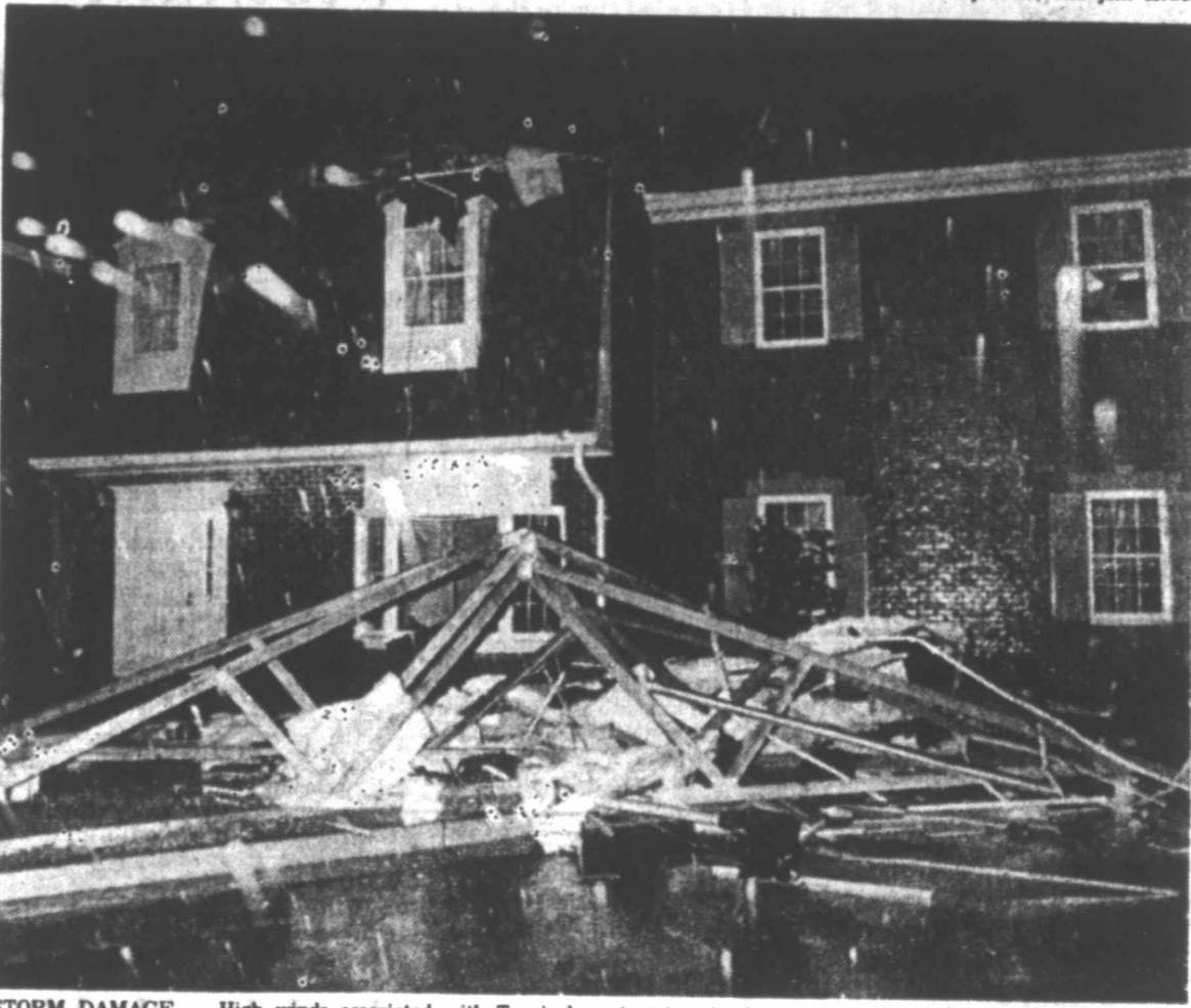
STORM DAMAGE — High winds associated with Tropical Storm David tore the roof from this house in Fairfax County, Va., Wednesday night. The storm ripped across northern Virginia, triggering heavy rains and flash flooding. Hundreds of persons in Maryland, most of them in Baltimore, had to flee their homes early today because of flooding. (AP Laserphoto)
