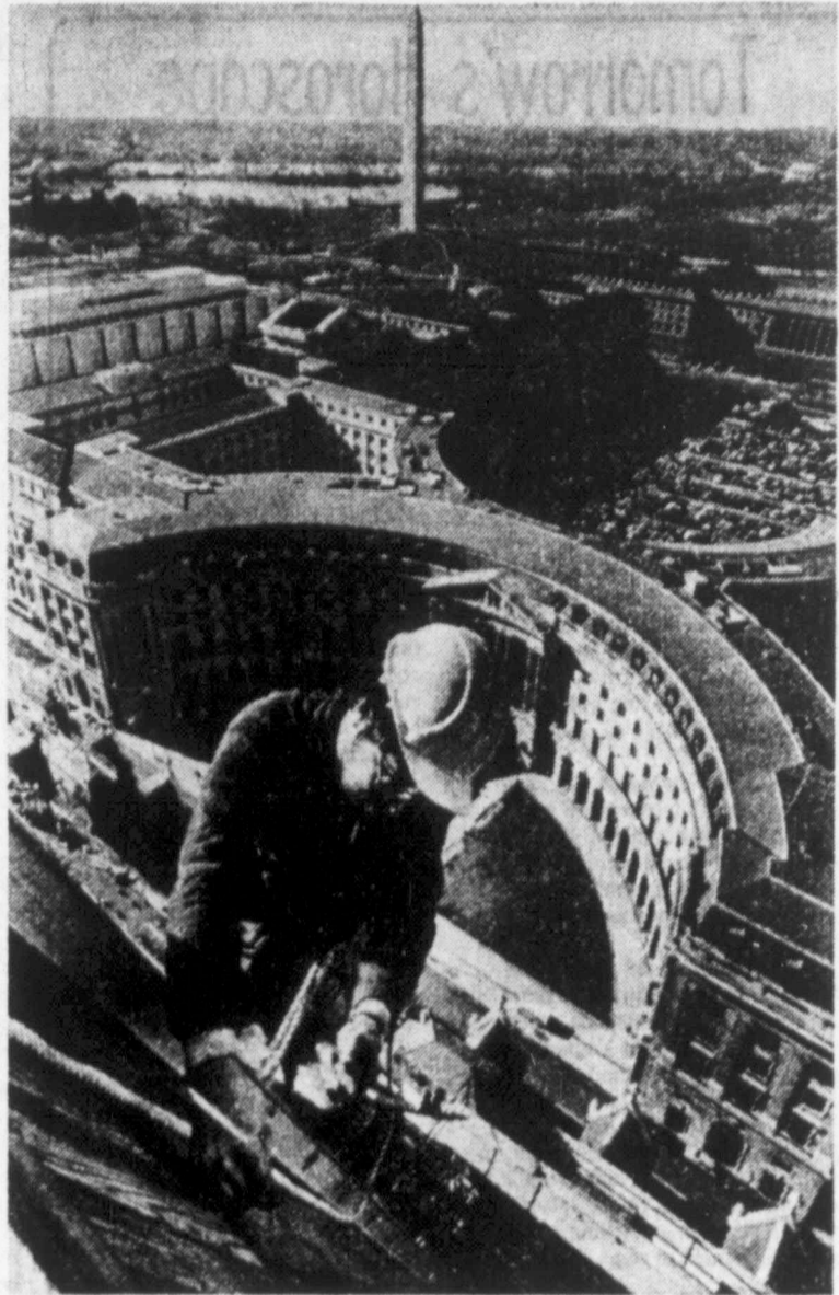
LONELY AT THE TOP — Slater Mike Bollinger of Baltimore hangs by a rope 315 feet above the street while working on the tower of the old Post Office in Washington, D.C., with the Washington Monument in the background. (AP Laserphoto)
