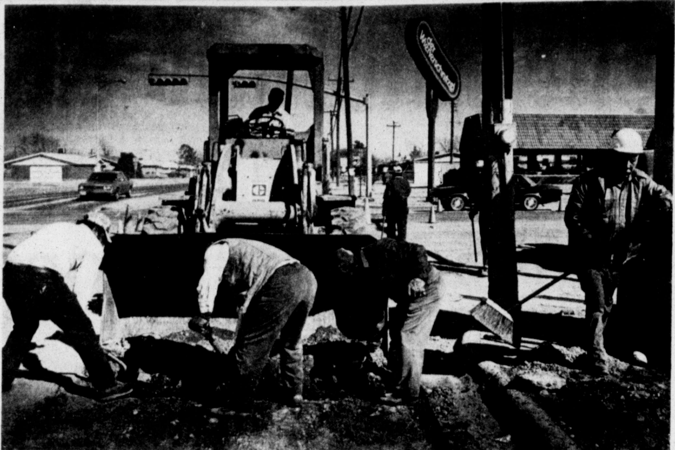
Workmen prepare to pave a section of Illinois Avenue that had been dug up for placement of a utility line.
