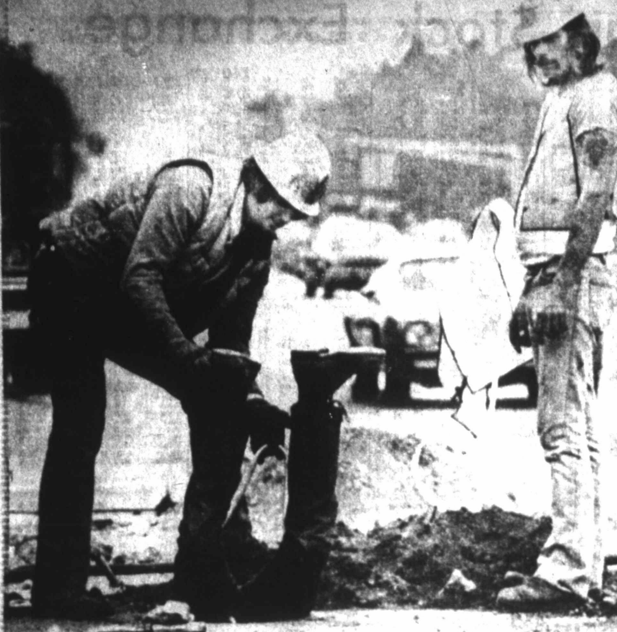
The legs of construction worker Steve Gieryn, center of New Bedford, Mass. are all that's visible of him as he takes the head-first approach to repairing an exca-
