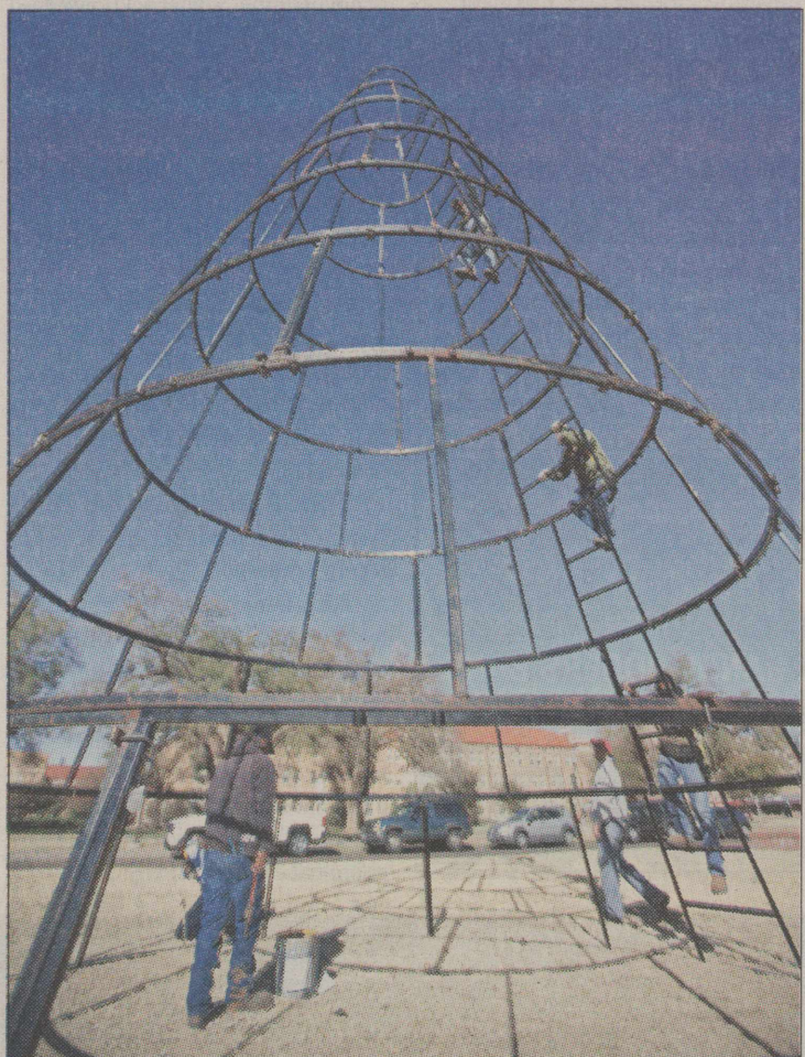
PHOTO BY ISAAC VILLALOBOS/The Daily Toreador CONSTRUCTION BEGINS ON the Christmas tree Tuesday located on the lawn behind the Texas Tech University seal. The Christmas tree is included in the annual Carol of the Lights ceremony, which will be hosted Dec. 1.
