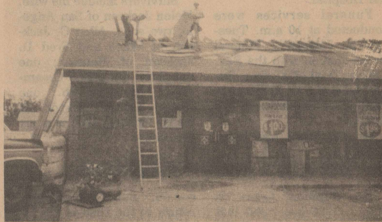
WORKMEN ATOP THE Town and Country Store in Bronte are working to cover the gaping hole left by a midnight fire on Monday. The blaze was quickly brought under control by the Bronte VFD and damage was mostly limited to the attic and roof.
