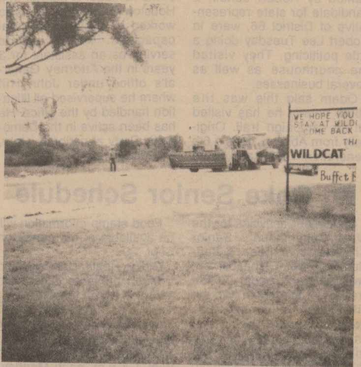
PAVERS PUT DOWN final asphalt layer on the road leading to Wildcat Marina and Lake Spence on Tuesday.
