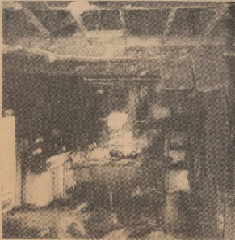
The family home of County Commissioner James A. and Brenda Tidwell of Bronte was a near total loss due to fire last Wednesday night. The top photo showing the exterior of the home, displays little of the extensive damage that shelled the interior of the structure (bottom photo). Lightning was listed as the probable cause of the fire.
