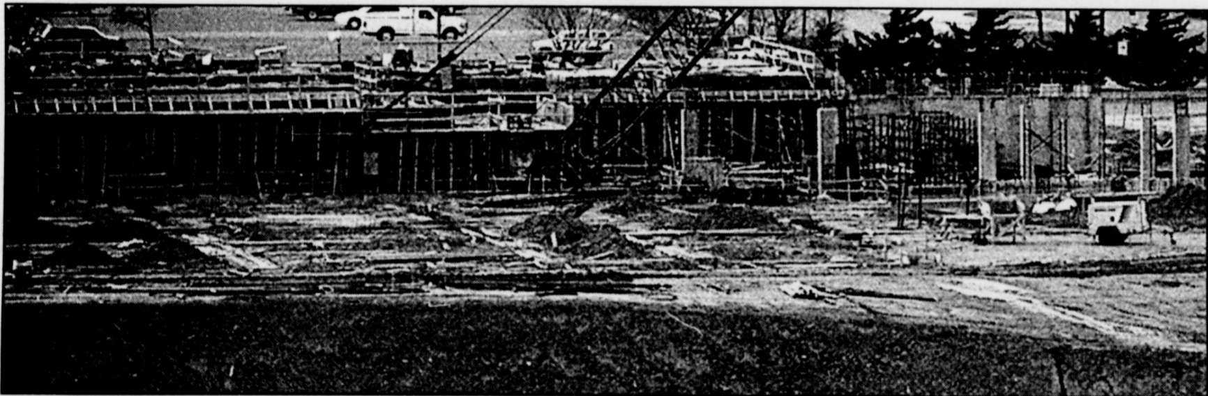
Slowly but surely: Construction of the United Spirit Arena will cost about $52 million.
