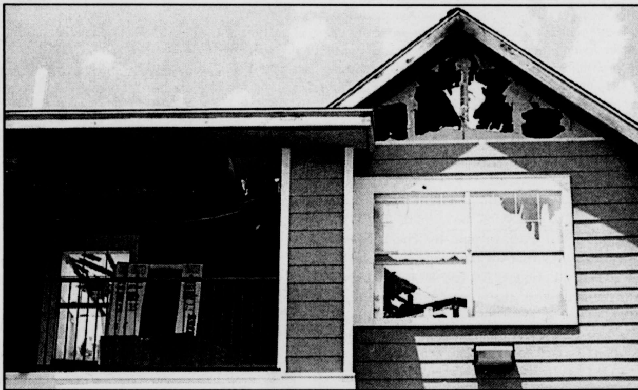
Cleaning Up: A fire in an attic Tuesday in one part of the Jefferson Commons apartment complex at 1002 Frankford Ave. caused around $700,000 worth of damage. The complex will be composed of 80 percent Tech students in the fall.
